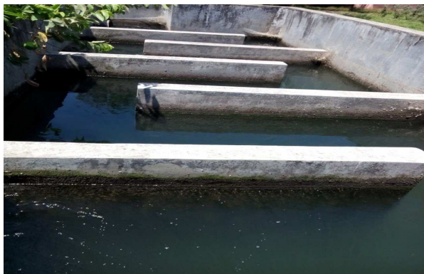
Plate-2 Showing sampling site-2 (Outlet of 18 MLD STP)
